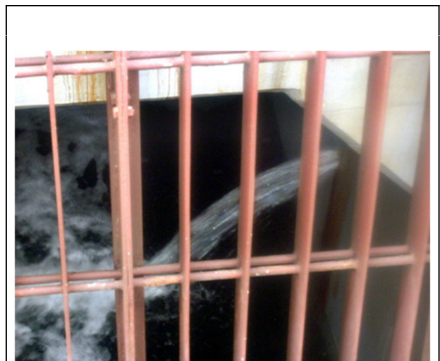
Radioactive water leaks into the sea April 2 from a crack in a pit wall near the water intake of the No. 2 reactor at the Fukushima No. 1 nuclear power plant. (TEPCO)
