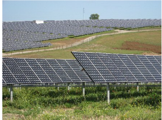
A solar power generation facility
