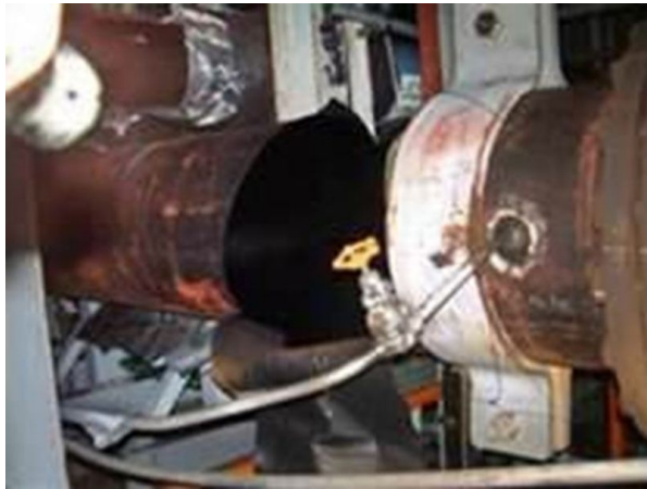
Pipes at aging Mihama reactor ruptured, releasing steam that killed four and injured seven in 2004
