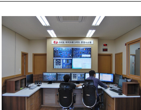
Gasa Island Microgrid Control Centre: Courtesy of KEPCO.
