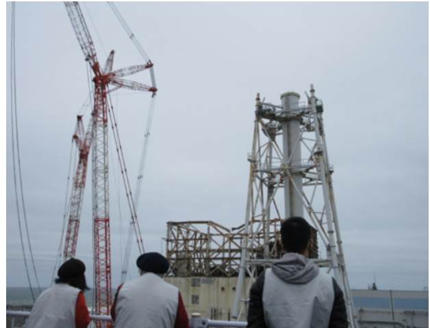
Reactor 1 at Fukushima Daiichi Nuclear Power Plant April 16, 2022. Credit: TEPCO
