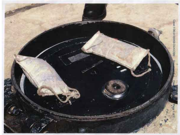
Entrance hatch to the silo used for maintenance. The peace activists used hammers to make the dial lock unusable.
