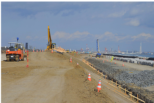
Seawall construction in Sendai, in Miyagi Prefecture, which was hard-hit by the 2011 tsunami. Conservationists and some scientists say the Japanese government could be doing far more to sustainably rebuild its coastal storm defenses, including constructing seawalls further inland, where they won't fragment marshes, dunes, tidal flats, and beaches. (Photo by Winifred Bird)
