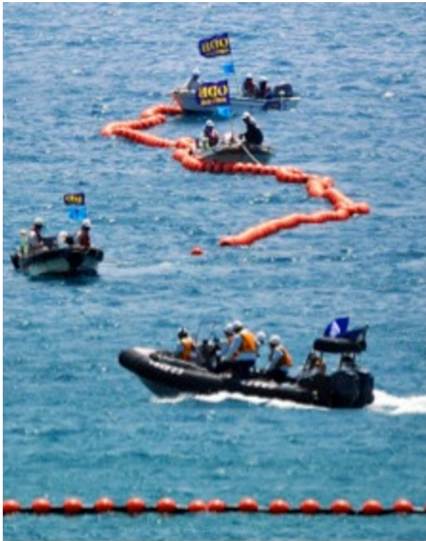
Coastguard rubber speed boats protecting the laying of a floating barricade by Okinawa Defense Bureau work teams, Henoko, 14 August 2014 (photo: Okinawa taimusu )
