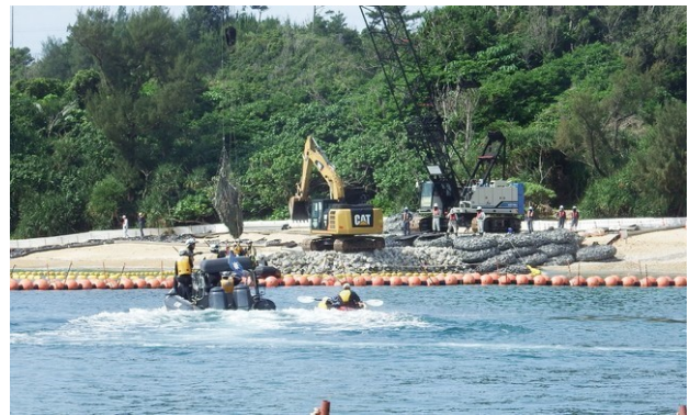
A protester on a kayak approaches Henoko construction site, May 15, 2017. Photo: Tsuyoshi Kitaueda
