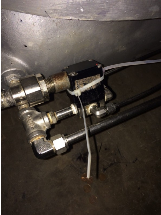
Photo from an inside source reveals the solenoid bypass which led to the June 2016 leak
