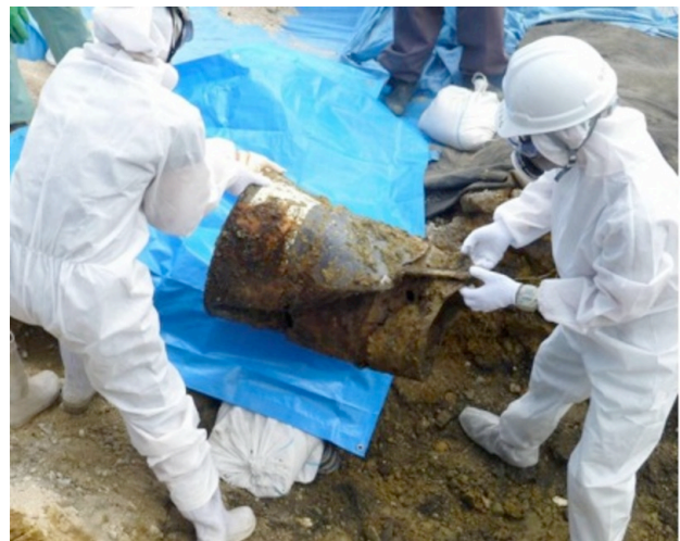
Workers unearth the barrels discovered beneath a soccer pitch in Okinawa, City.
