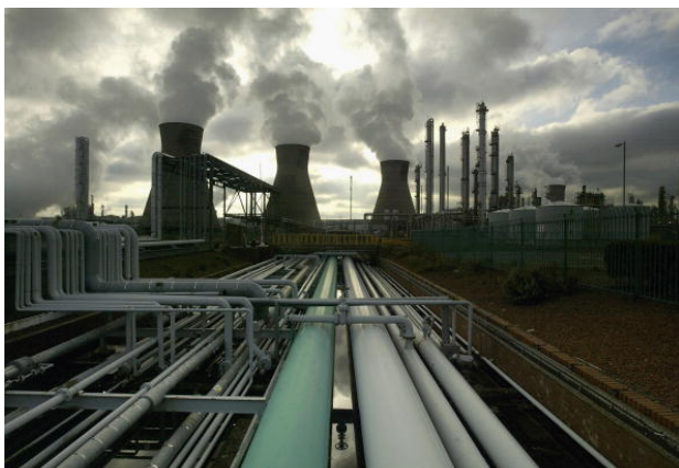
A Syrian Oil Facility
