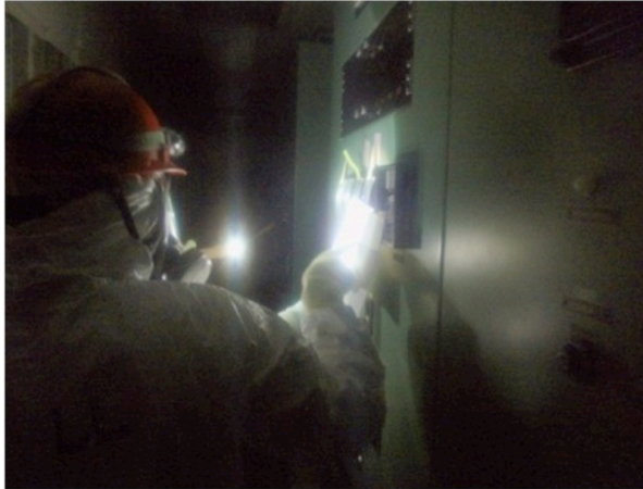
In this photo released by Nuclear and Industrial Safety Agency, a TEPCO worker looks at gauges in the control room for Unit 1 and Unit 2 at the tsunami-crippled Fukushima Dai-ichi nuclear power plant on March 23, 2011.
