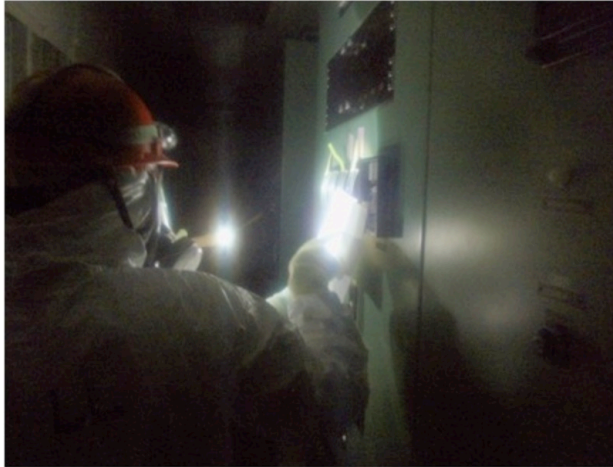
In this photo released by Nuclear and Industrial Safety Agency, a TEPCO worker looks at gauges in the control room for Unit 1 and Unit 2 at the tsunami-crippled Fukushima Dai-ichi nuclear power plant on March 23, 2011.
