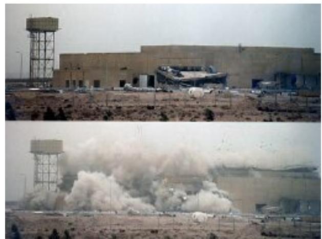
" 'Before and After': the destruction of a building at Al Atheer in the summer of 1992 carried out under the supervision of an IAEA Inspection team. The building had been used for Iraq's secret nuclear weapons programme. (Al-Atheer, Iraq, 1991-1998)." Action Team 1991-1998/IAEA
