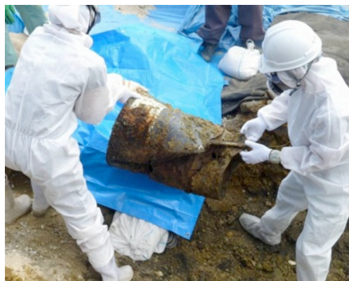
Workers unearth the barrels discovered beneath a soccer pitch in Okinawa, City.
