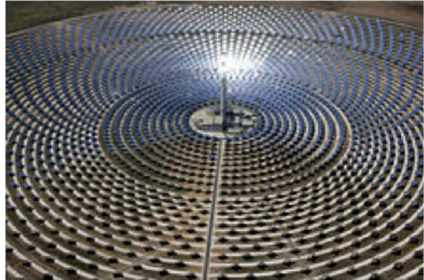
Fig. 7. Gemasolar power tower plant in Spain
