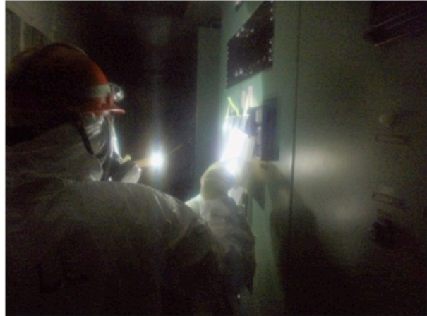
In this photo released by Nuclear and Industrial Safety Agency, a TEPCO worker looks at gauges in the control room for Unit 1 and Unit 2 at the tsunami-crippled Fukushima Dai-ichi nuclear power plant on March 23, 2011.
