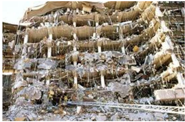
On April 19, 1995, the Alfred P. Murrah Federal Building was bombed, killing 168 and injuring 800.
