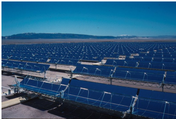
Dunhuang Solar Plant
