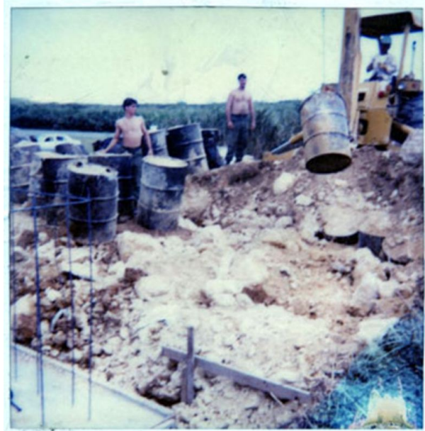
Deep deception: The worksite where Kris Roberts unearthed over 100 leaking barrels is seen in a photo taken in summer 1981. KRIS ROBERTS
