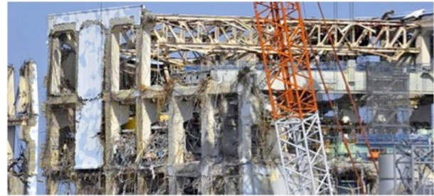
Reactor # 4 at Fukushima Daiichi
