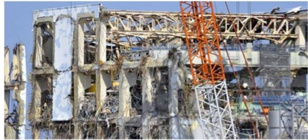
Reactor # 4 at Fukushima Daiichi
