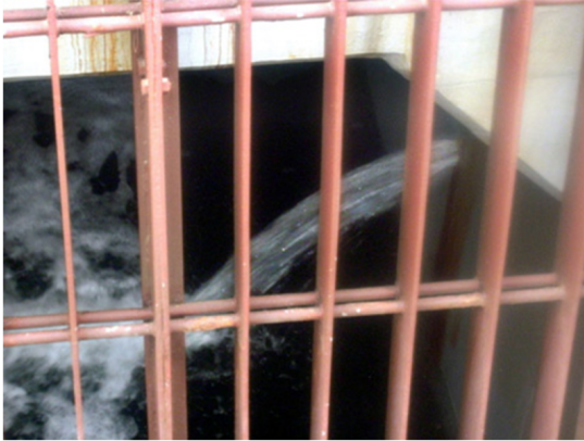
Radioactive water leaks into the sea April 2 from a crack in a pit wall near the water intake of the No. 2 reactor at the Fukushima No. 1 nuclear power plant. (TEPCO)
