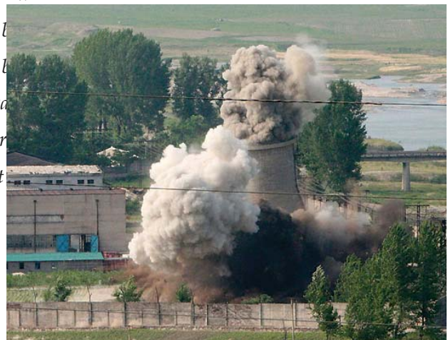
Cooling tower explodes at Yongbyon
