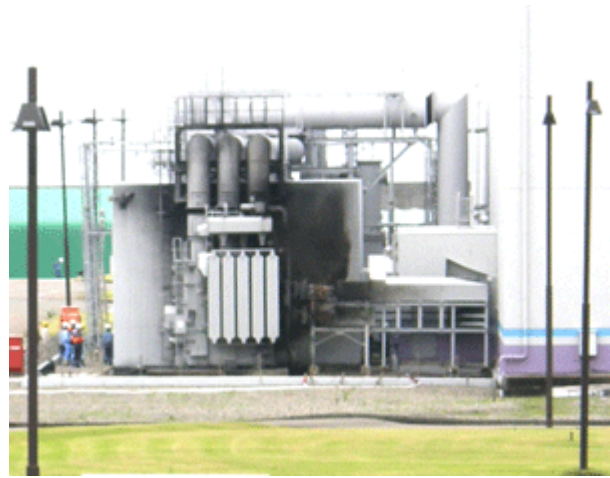
Burnt out transformer at the plant
