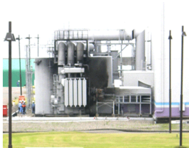
Burnt out transformer at the plant
