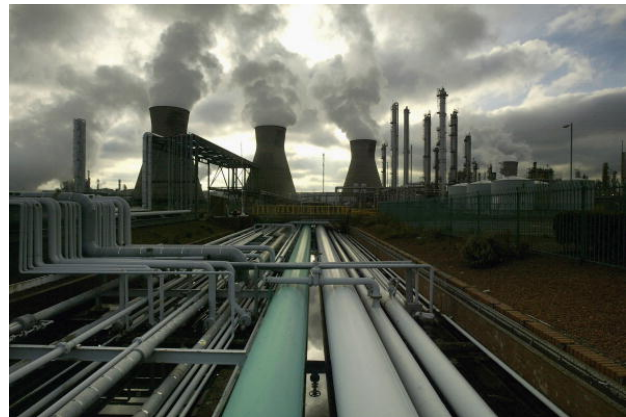
A Syrian Oil Facility
