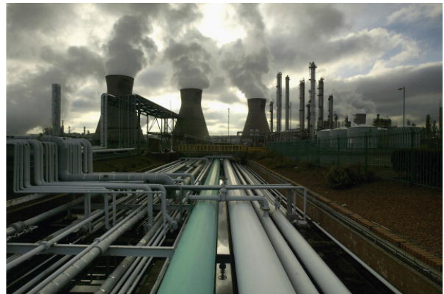
A Syrian Oil Facility
