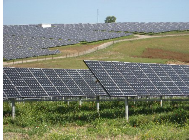
A solar power generation facility
