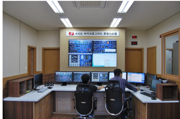
Gasa Island Microgrid Control Centre: Courtesy of KEPCO.
